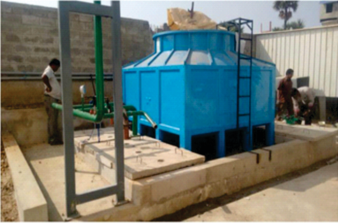
M/S Shree Motherplast Pvt Ltd (Vallam-Chennai) Cooling Tower
