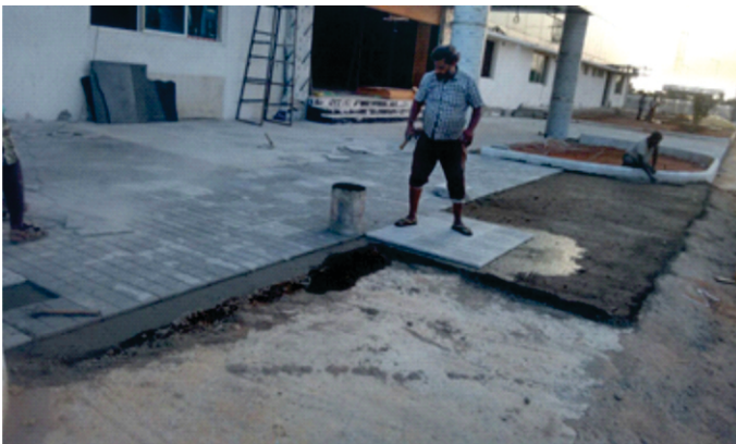
M/S Asian Sealing Products Pvt Ltd (Pillaiakkam-Chennai) Entrance Portico Tile Laying Work
